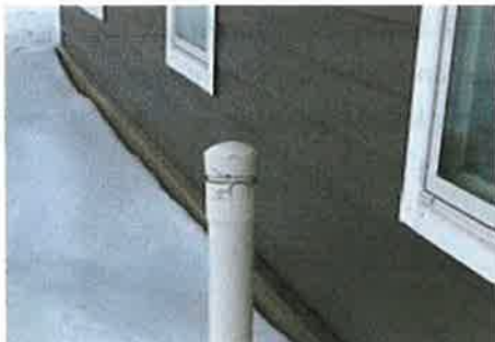
Sewer line not in us. This is not for this home
