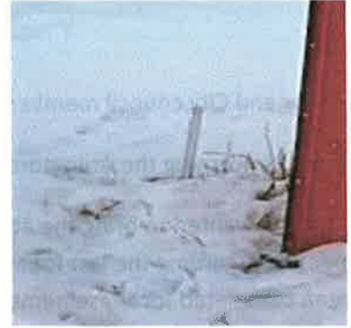
curb stop not in use
