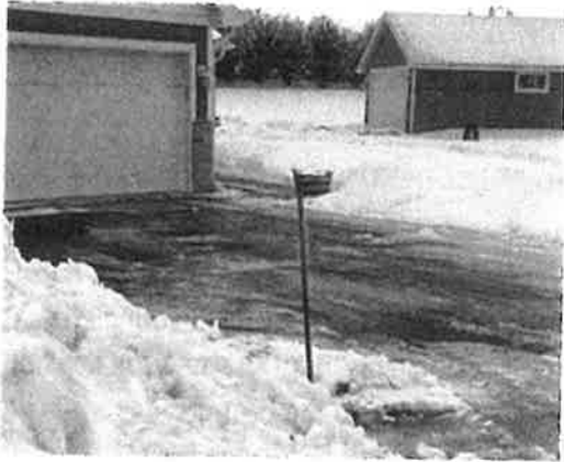
curb stops in use. Some are 2 feet below grade
