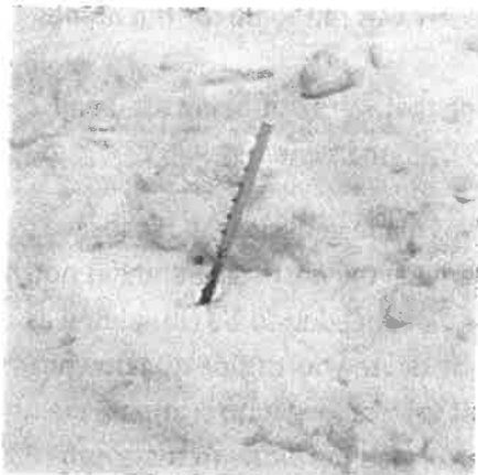
curb stop not in use
