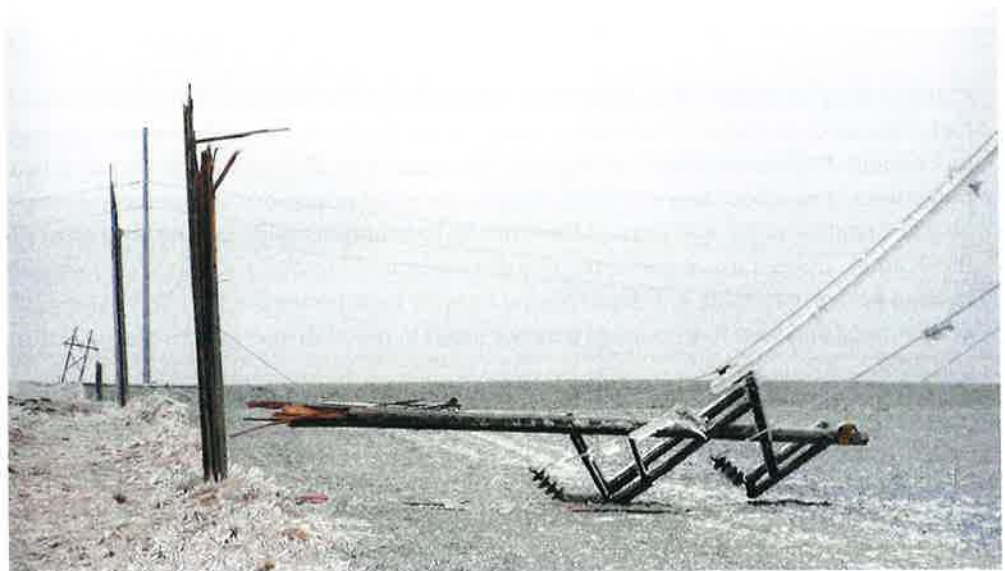
Powerlines down in Worthington, Minnesota (Mark Steil, 2013)
