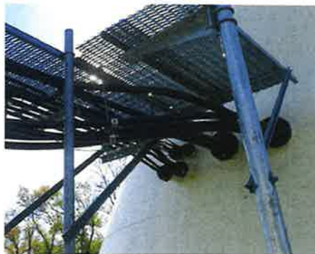
3 COAX TO TOWER PHOTO
