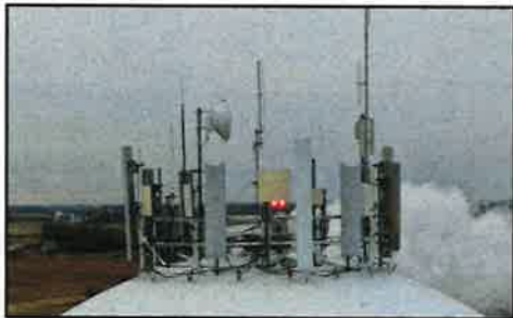
4 'Z' SECTOR ANTENNA MOUNT PHOTO SCALE: NONE
