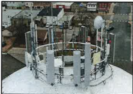
3 'Y' SECTOR ANTENNA MOUNT PHOTO SCALE: NONE
