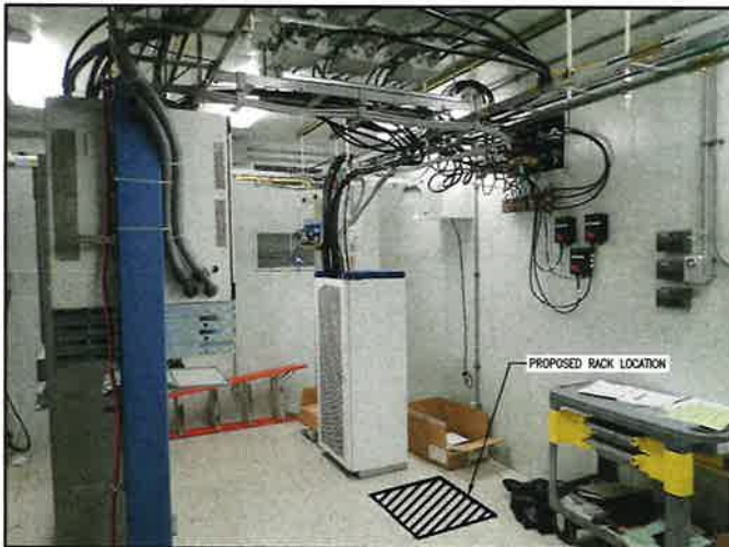
4 LTE CABINET PHOTO
