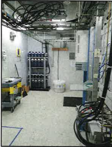
1 OVERALL SHELTER INTERIOR PHOTO
