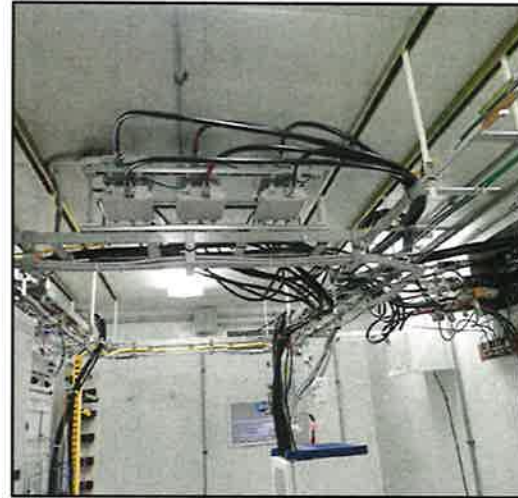
3 CABLE TRAY PHOTO
